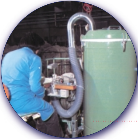
Fixed installation on textile cutting machine.
